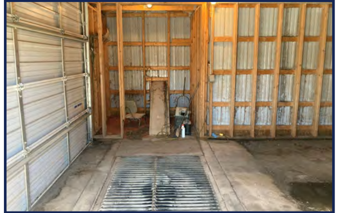
Indoor Receiving Pit
