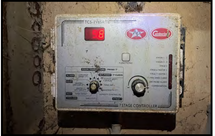
Gestation Room Controller
