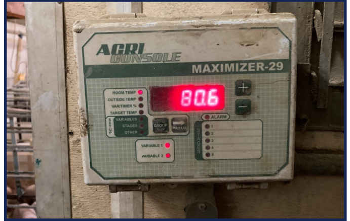
Farrow Room Controller
