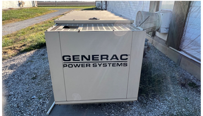
Natural Gas Generator
