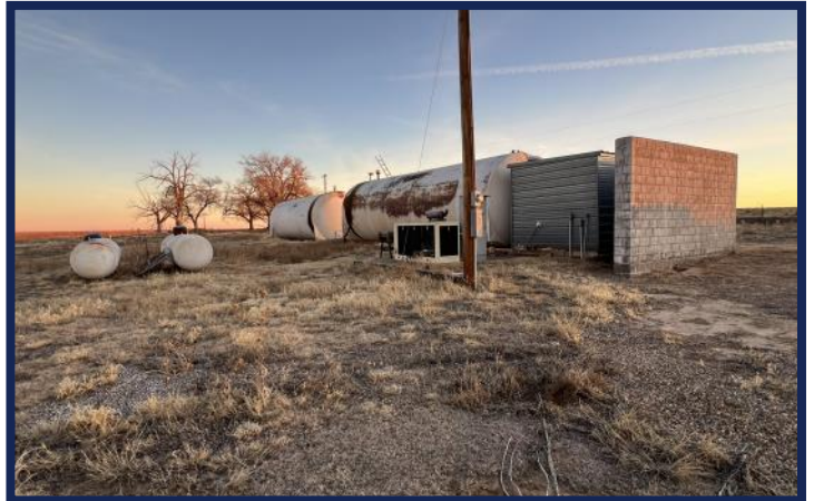
Water Tank & Standby Generator—North Farm
