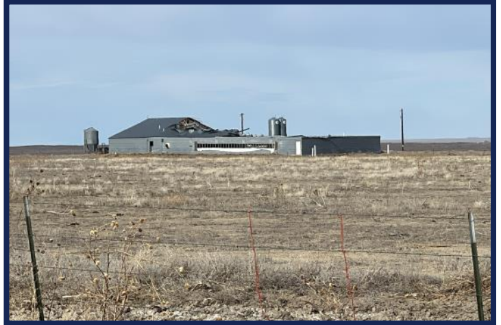
Isolation - Roof, Rafters & Ceiling need Replaced
