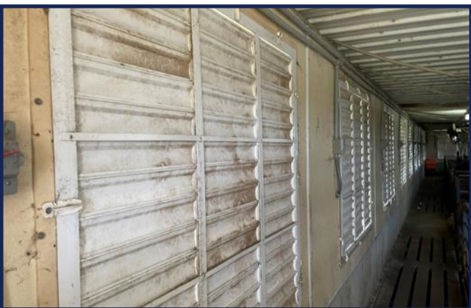
Bank of Fans North Wall Gestation Building
