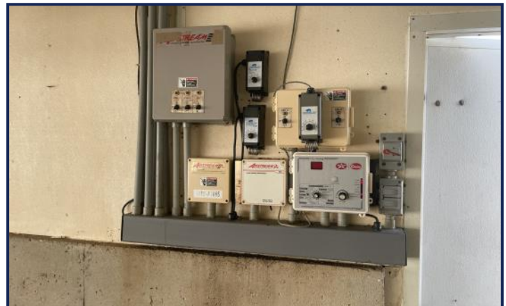
Ventilation System 2000 Barn
