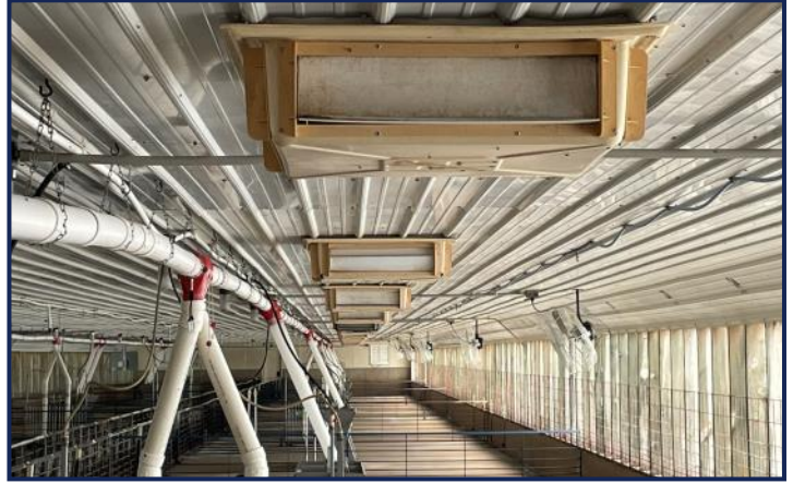
Ceiling Inlet 2000 Barns
