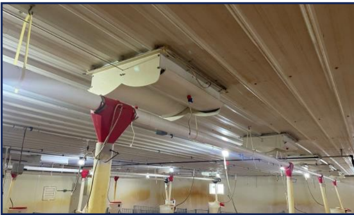
Actuated Inlet - Rooms 9 & 10
