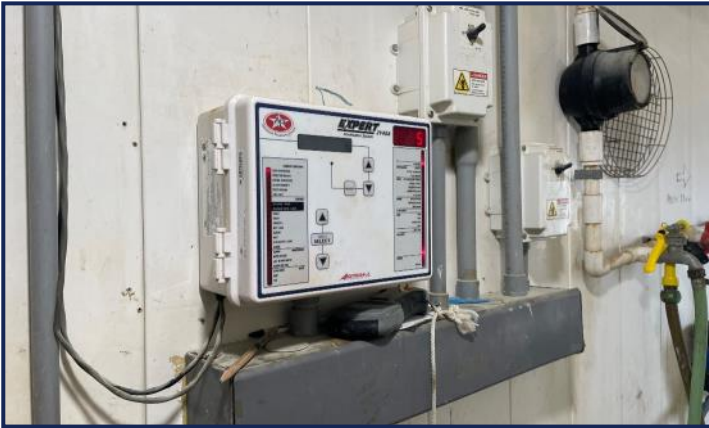
Typical Ventilation Controller
