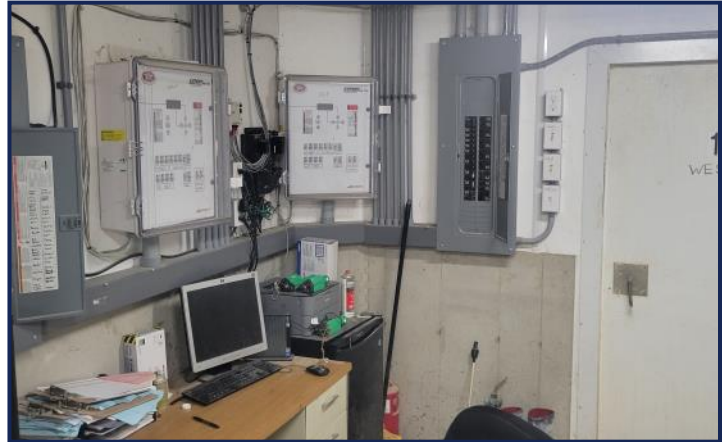
Controllers and Alarm
