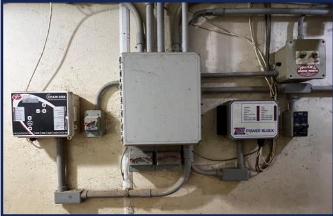
Room Controller East Rooms
