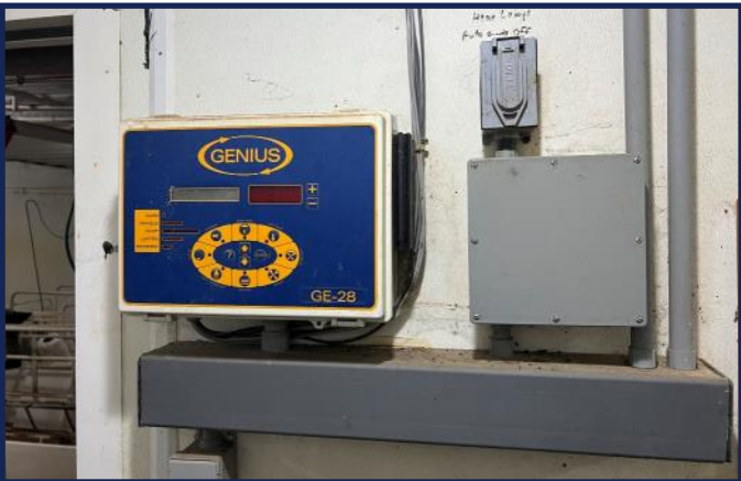
Farrow Room Controller West
