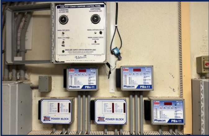
Room Controller East Gestation
