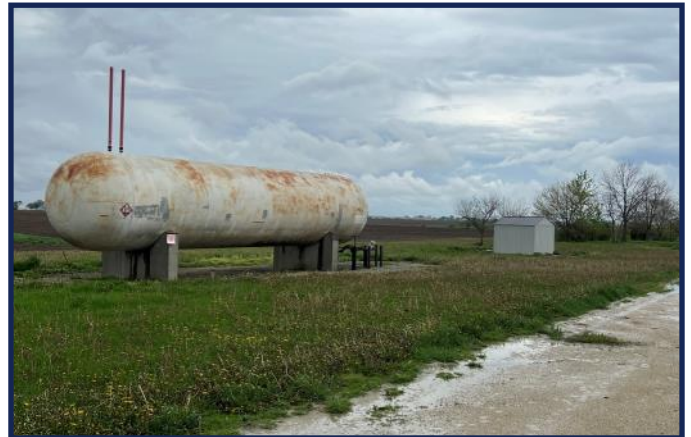
Site 18000 Gallon LP Tank
